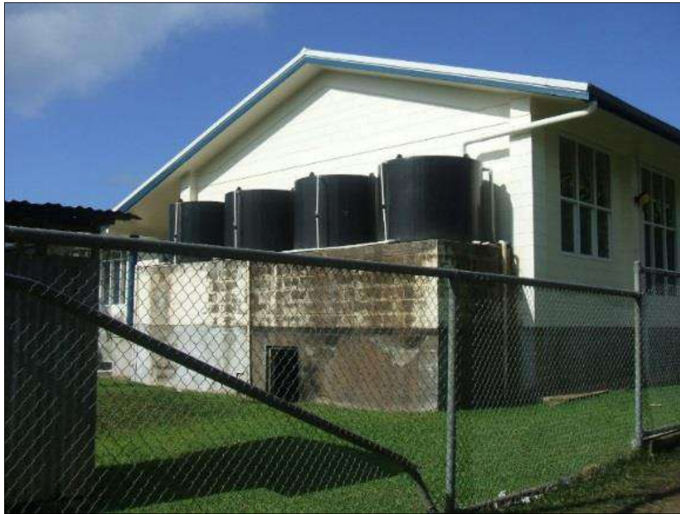
Figure 6.6: Water tanks at the Latter Day Saints church compound at Maagiagi.
